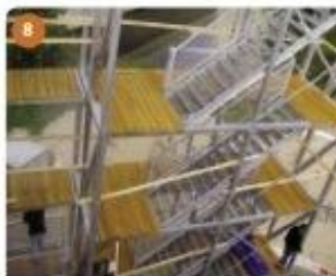
8 Staircases designed tailor made for each project;
