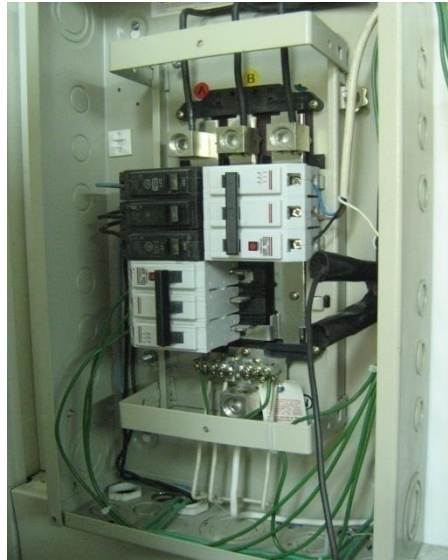
Figura A 53. Tablero Normal #08 E-105
