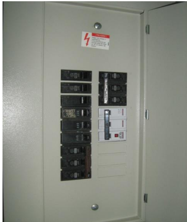
Figura A 39. Tablero normal #10 Laboratorio de Control
