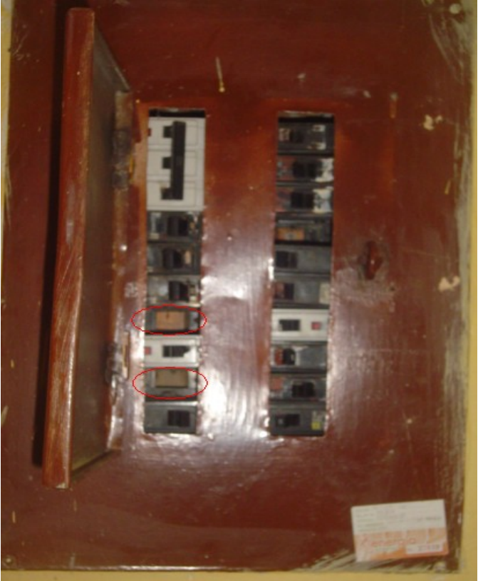
Figura 9. Tablero principal B.
