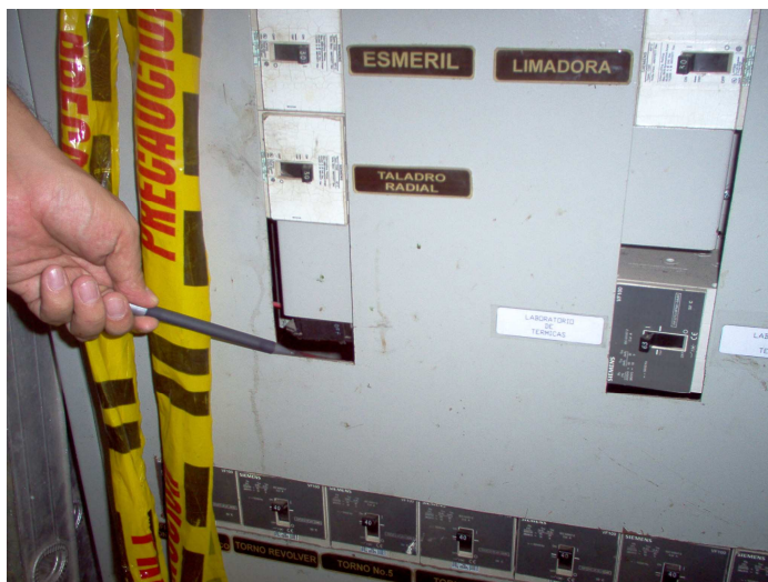
Figura 17. Tablero Taller Principal (abertura 1)
