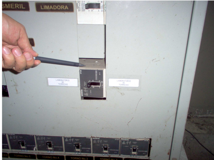
Figura 18. Tablero Taller Principal (abertura 2)
