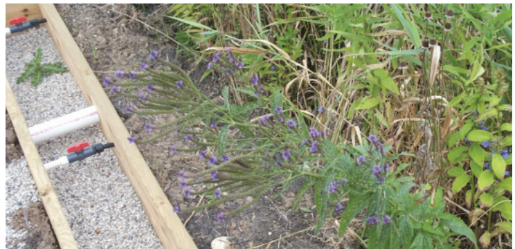
A close up of the line that carries oxygen generated by the windmill to the appropriate bacteria tank. Some of the wildflowers on site can also be seen in this photo. Photo courtesy of Tom Mellon.
