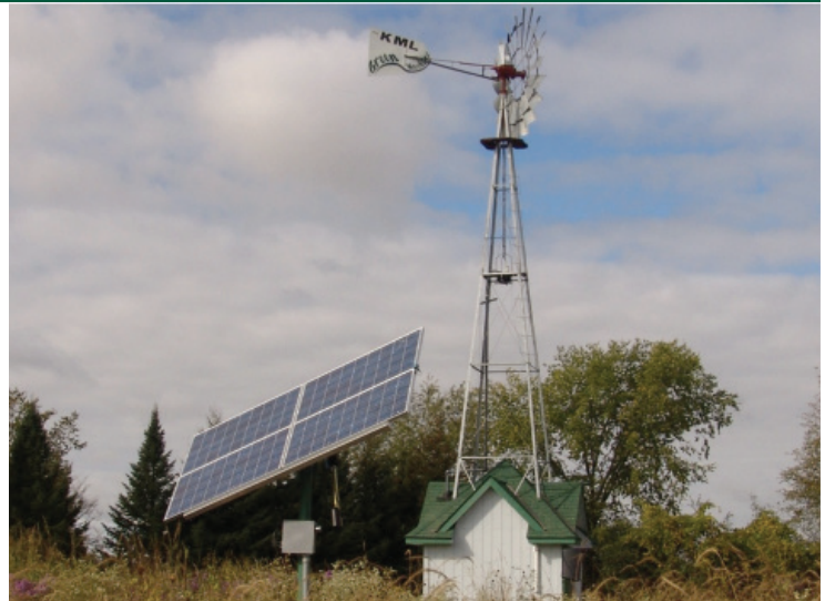
A windmill and solar panel stand in the constructed wetland. The solar panel provides power to run monitoring equipment, while the windmill aerates the aerobic bacteria tank that processes the effluent. Photo courtesy of Tom Mellon.
