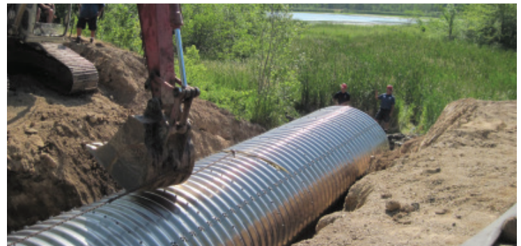
The Ozaukee County Highway Department installs a fish passage culvert near Daly Lake on the Riveredge Creek. Shady Lane Road crosses this creek, causing the need for the culvert. Photo courtesy of the Ozaukee County Planning and Parks Department.
