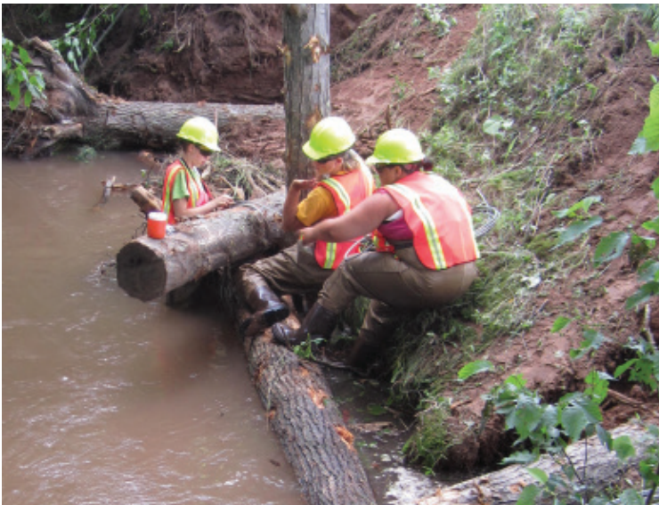
Workers position a log in the stream channel, which will help prevent sedimentation and provide habitat for fish and wildlife. Photo courtesy of Inter-Fluve, Inc.
