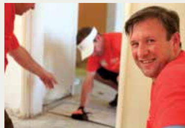
Corporations can encourage civic engagement like The Home Depot's partnership with Habitat for Humanity where volunteers from the company's vendors build a home.
