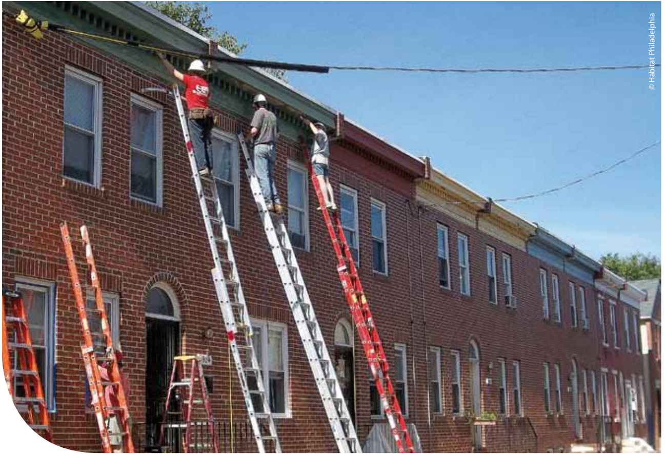
Oak's partner Habitat for Humanity Philadelphia aims to carry out "whole block" repairs to Philadelphia's ageing housing stock. This grant was approved to run over four years, from 2011 to 2015.
