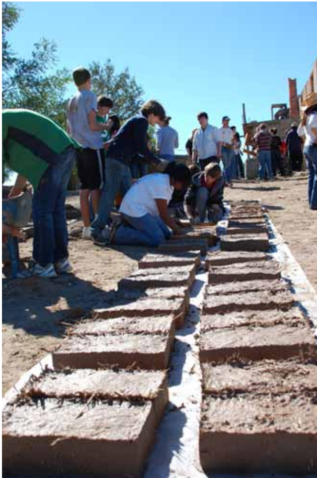
Youth making bricks at an on-site historical preservation project. Courtesy of Cornerstone Community Partnerships and photographer Anna Rutins.
