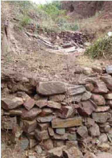
A check dam slows water from flowing down a gully and taking topsoil with it, and it increases water infiltration into the soil. Paul Hebert for CRS.
