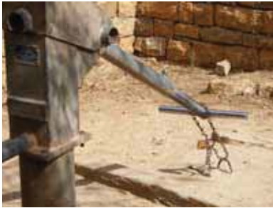
A community-managed hand pump in Adidaero is chained to prevent overuse, as there are still not enough water points for the population. The pump was open two hours each morning and afternoon. Paul Hebert for CRS.
