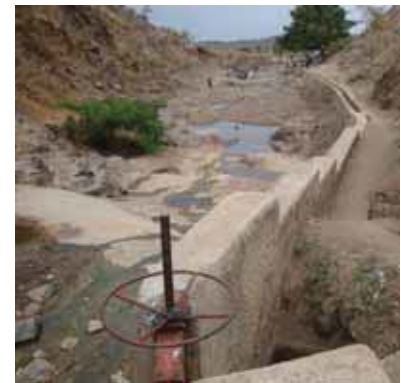
Harbu expensive irrigation structure. Tsegahun Tessema for CRS.
