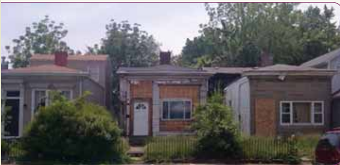
Before NSP funding: Vacant homes on East St. Catherine Street in the Shelby Park Neighborhood.
