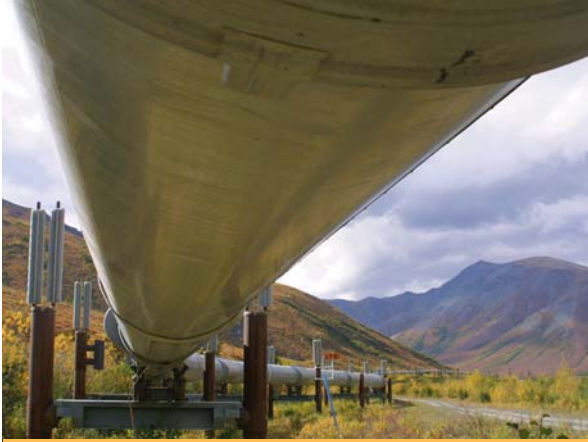
The Trans-Alaska Pipeline stretches 800 miles across the tundra and feeds 900,000 barrels of oil a day to the lower 48 states.
