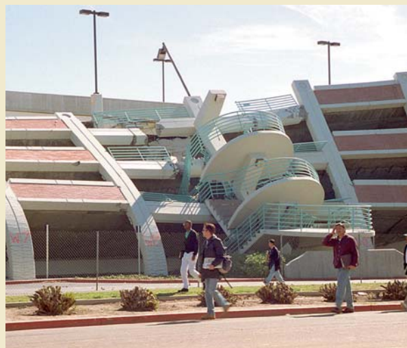
No parking: The 1994 Northridge earthquake toppled this campus garage.
