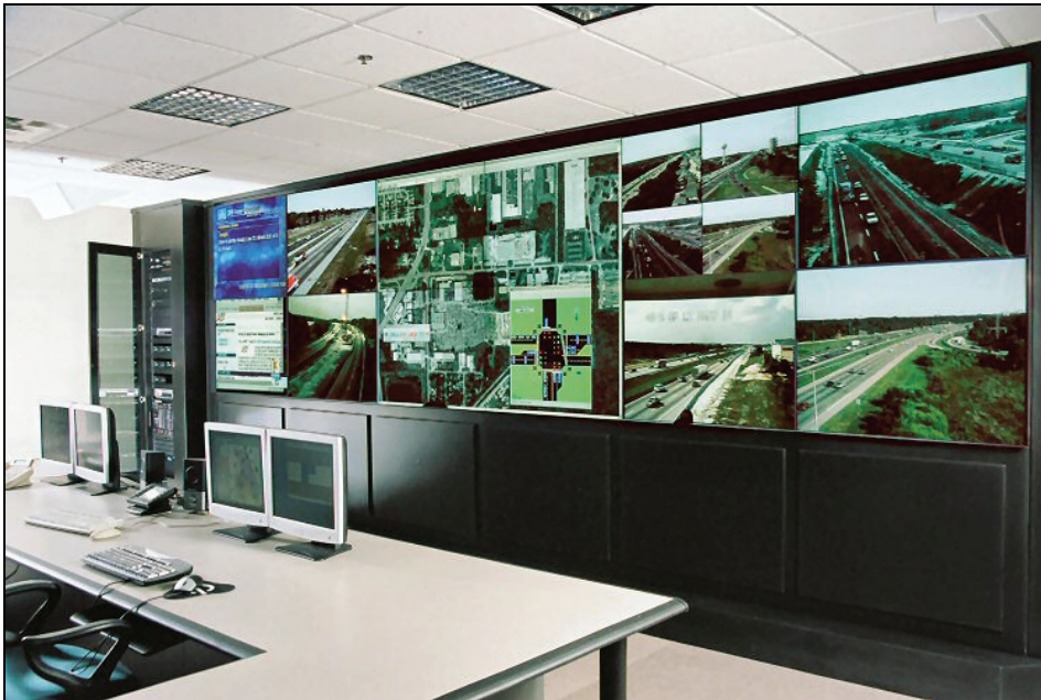
Figure 5: Seminole County Traffic Management Center
