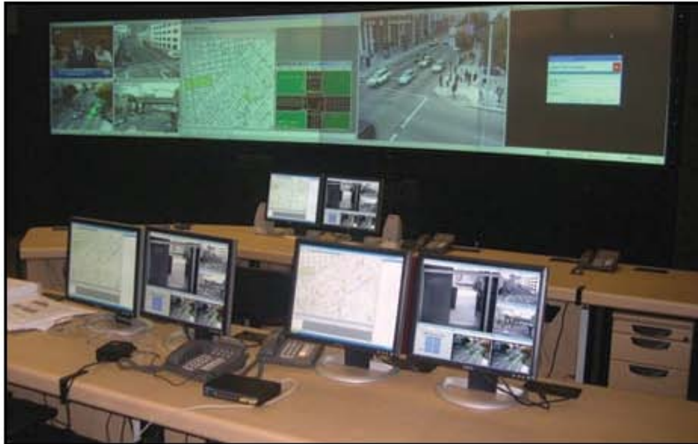
Figure 4: San Francisco Traffic Management Center
