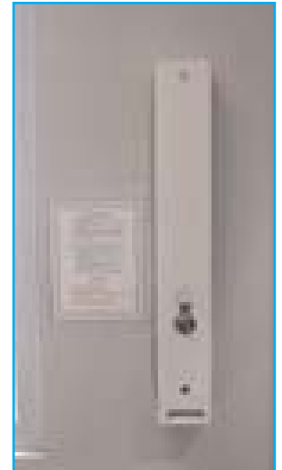
Condom dispensing machine installed (rules are posted to the left)
