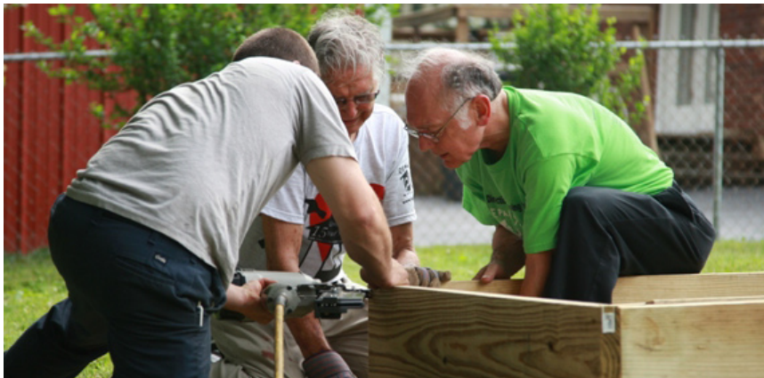
Volunteers work on an access ramp as part of New Directions' Repair Affair 2008.
