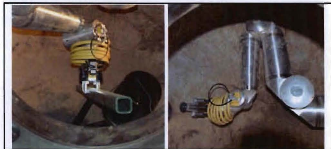
Figure 14. Cold testing of the sphere cleaning robotic system.
