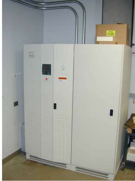
Figure 2. Installed Back-Up Power Supply System for Gradient Test Systems
