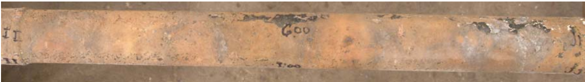
6 O'Clock – Opposite Gas Flow
