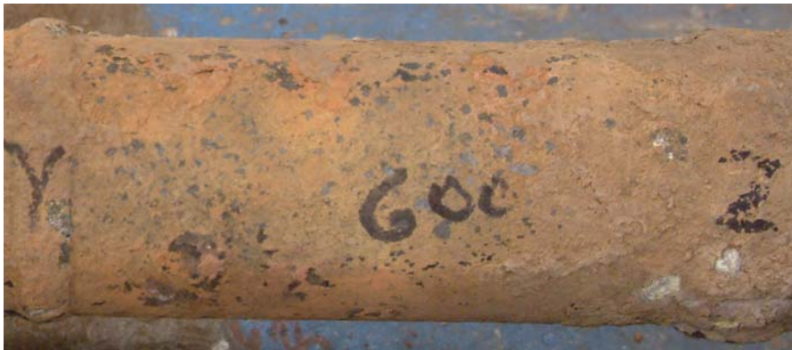
6 O'Clock – Opposite Gas Flow
