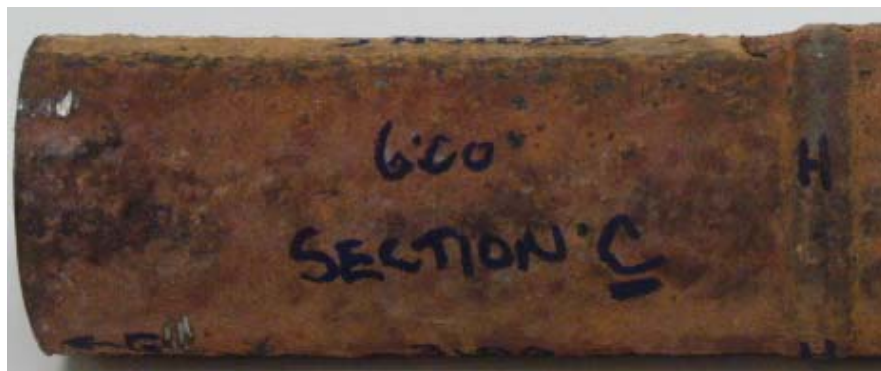
6 O'Clock – Opposite Gas Flow
