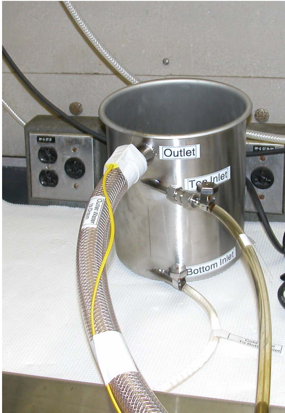
Figure 2-6. Portion of the second cooling water system.
