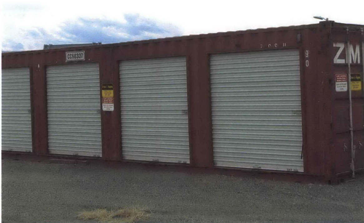
Doors added to the side of a Conex box. These may negatively impact the structural integrity of the box.
