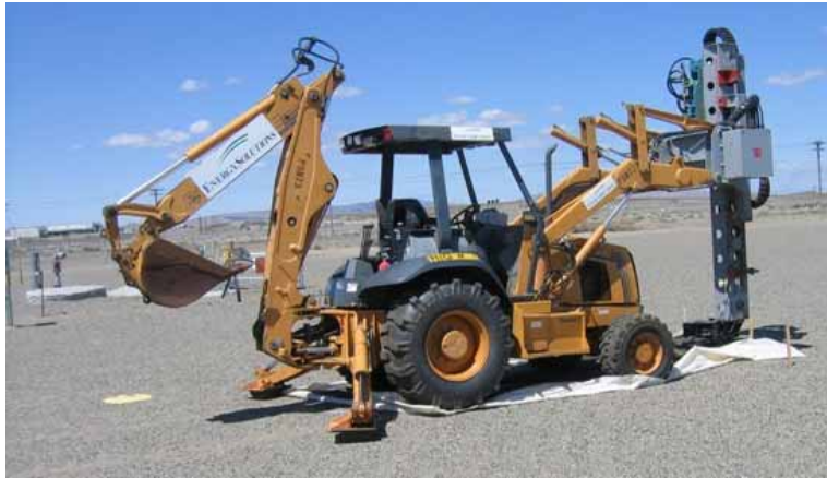
Figure 2.4. Hydraulic Hammer Used to Install Instruments in the T Tank Farm (Photo taken in the summer of 2006)
