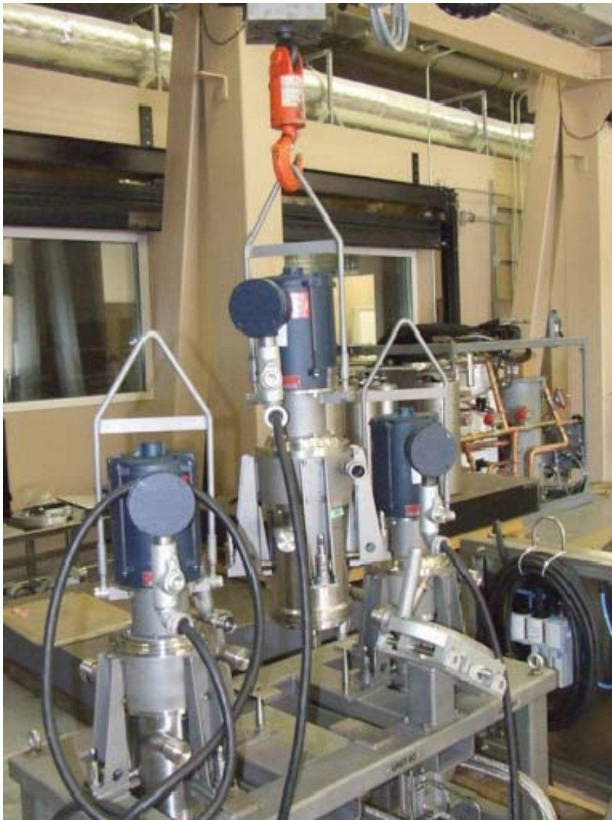
Figure 11 Removal of the middle unit with tapered locating pins visible on the frame
