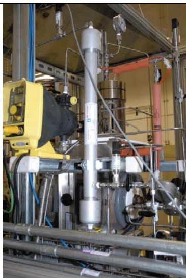
Figure 3.2n CO 2 separation reactor (metallic) and water injection pump (yellow).
