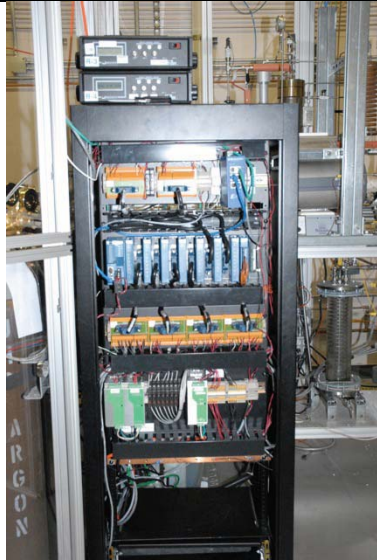
Figure 3.2e PLC panel for process monitoring and control.
