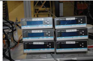
Figure 3.2i PID power controllers for band heaters, liquid product ceramic heaters, steam generator, and heat tracing.
