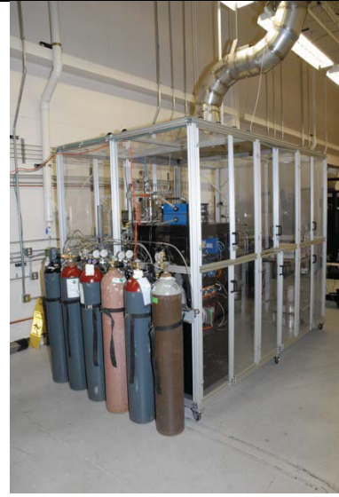
Figure 3.2g Compressed gas supply rack; enclosure custom exhaust duct.
