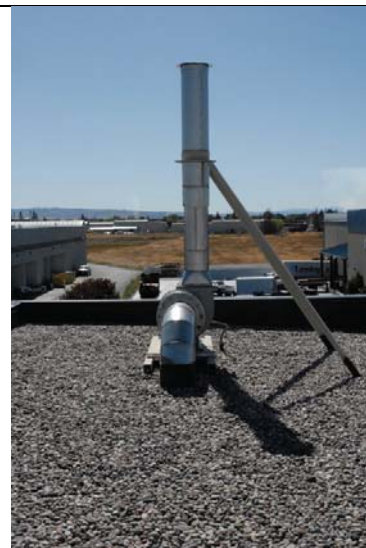
Figure 3.2d Variable frequency exhaust blower installed on BCTC Bay 9.
