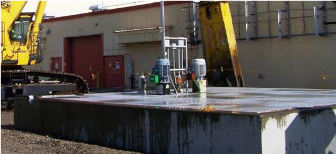
Figure 6. 183-NC Filter Backwash Sump.
