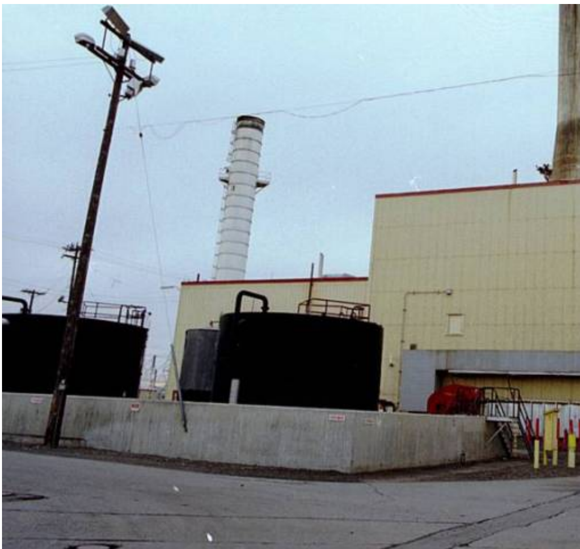
Figure 11. 184-ND Fuel/Diesel Oil Day Tanks.
