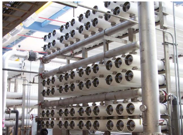
Figure 4. Spiral-wound membrane arrays in the El Paso, TX plant
