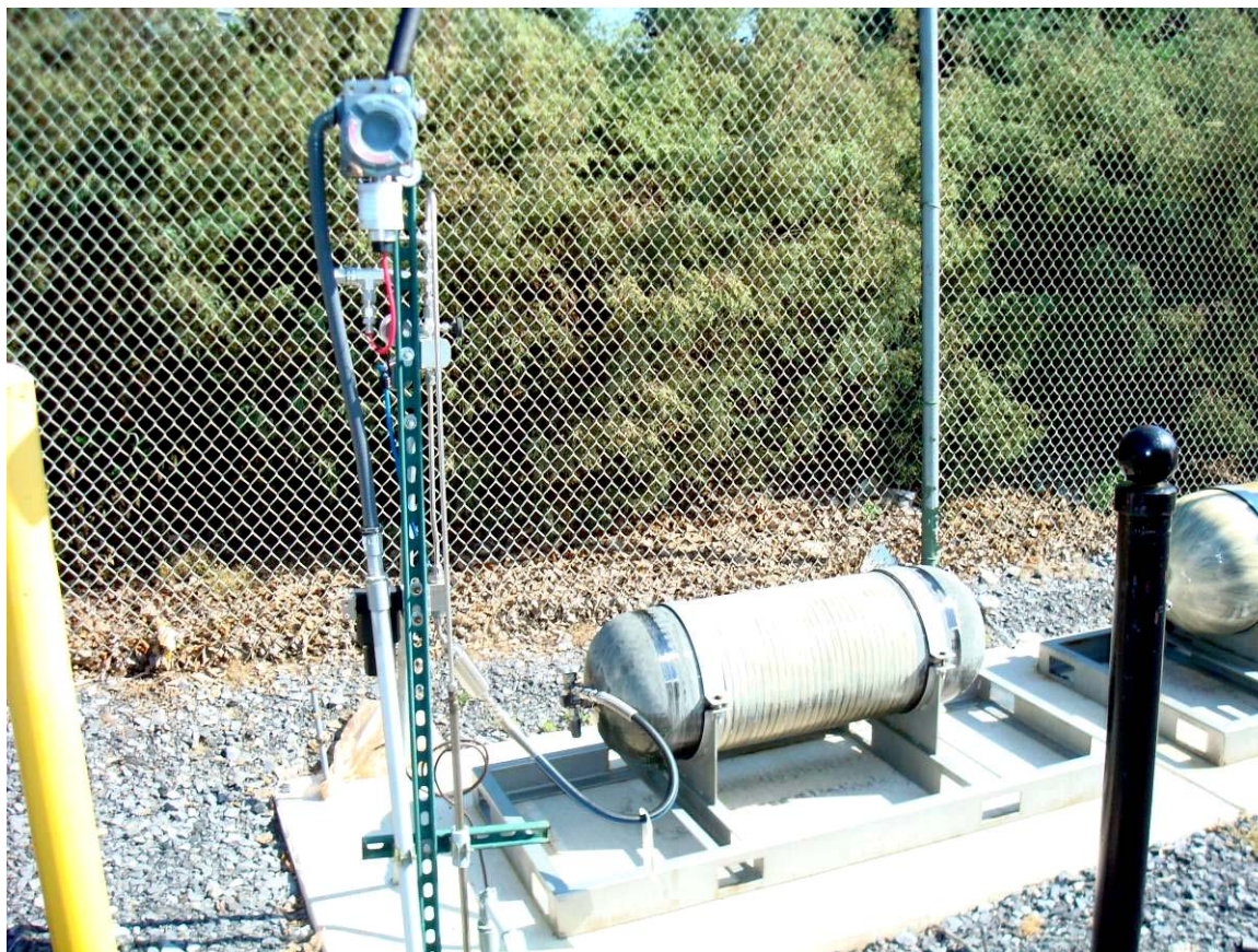
Figure 11: Gaseous Fuel Storage Tank, 3600 PSI
