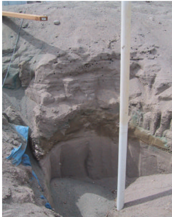
Figure 3.7. Wet Sill Observed West of the Dike and Adjacent to CPT-8 (Tube #5)
