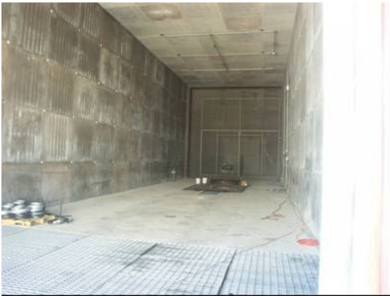
Figure 2: Internal view of XTF showing the air inlet (far end)
