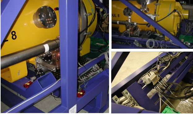
Figure 2: The installed instrumentation.
