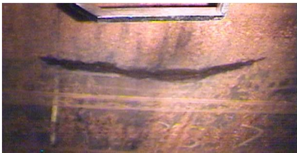
Figure 4. Example of through-wall bleedout.
