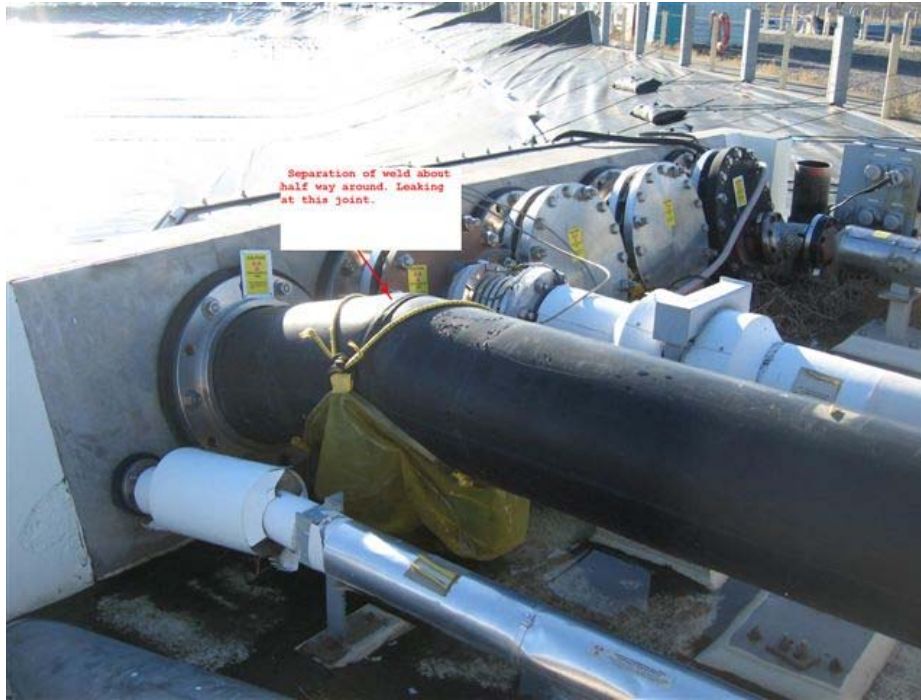
Fig. 1 – Location of bond failure on HDPE recirculation pipe
