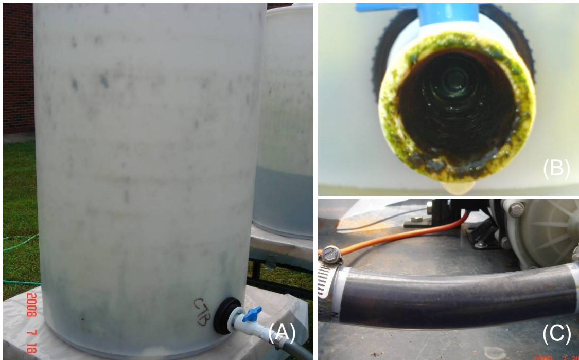
Figure D.19 Algae growth was observed in the cooling tower system – A) Makeup water tank B) Makeup water conduit C) Pump conduit. For future studies, it is recommended to wash the makeup water tank regularly to decrease the amount of algae released into the recirculating system.
