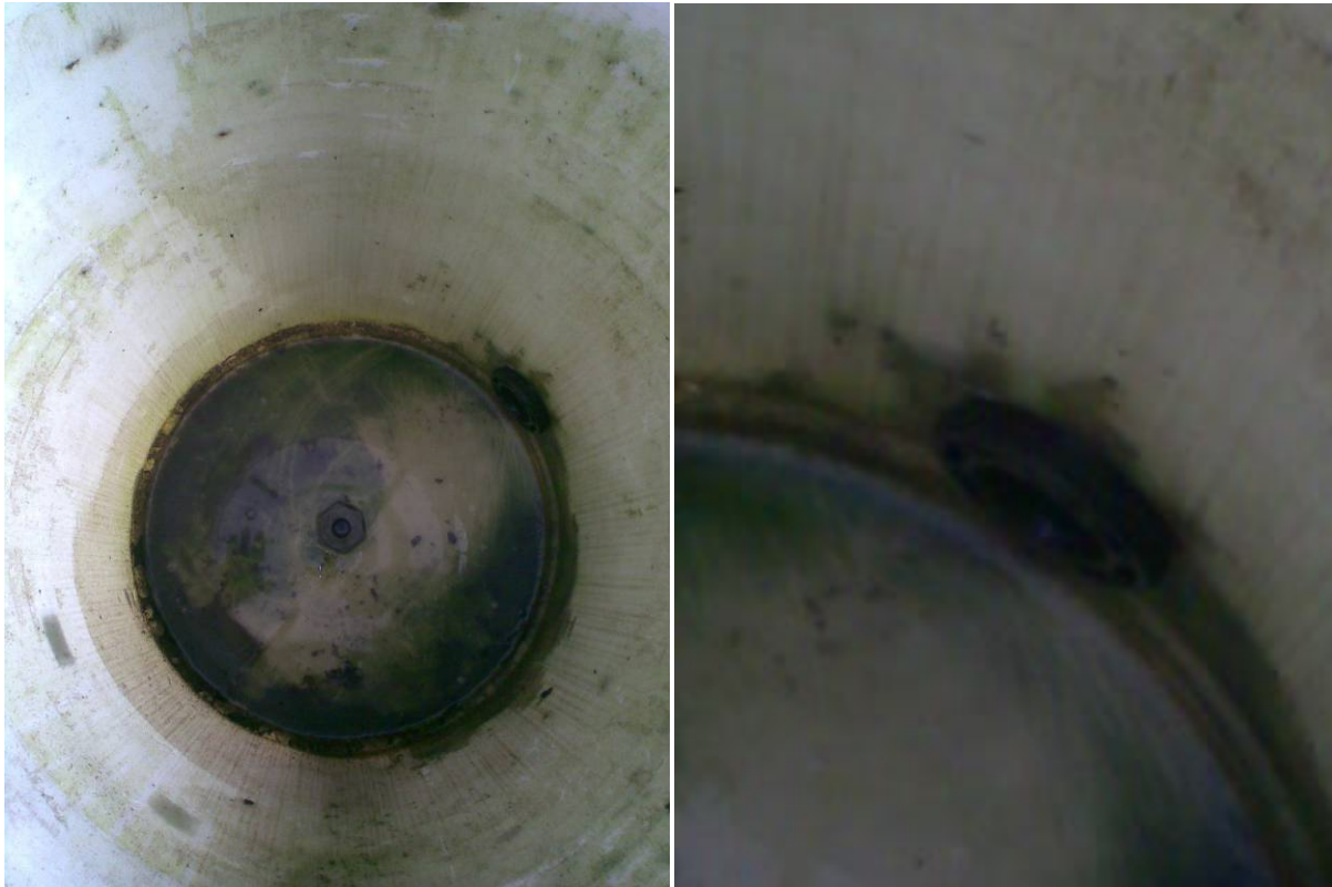
Figure D.24. Algae populated the bottom of the makeup water tank and near the through wall fitting. Since the tank was 44" height, we could only use long shaft brush to clean the bottom. After removing most visible algae, we disinfected the tanks with vinegar and low dosage of sodium hypochlorite in turns.
