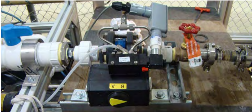
Figure 4.8. The Pneumatic Butterfly Control Valve Mounted Between Pump Skid and Tank Skid. The red throttle valve is also visible to the right of the butterfly valve.
