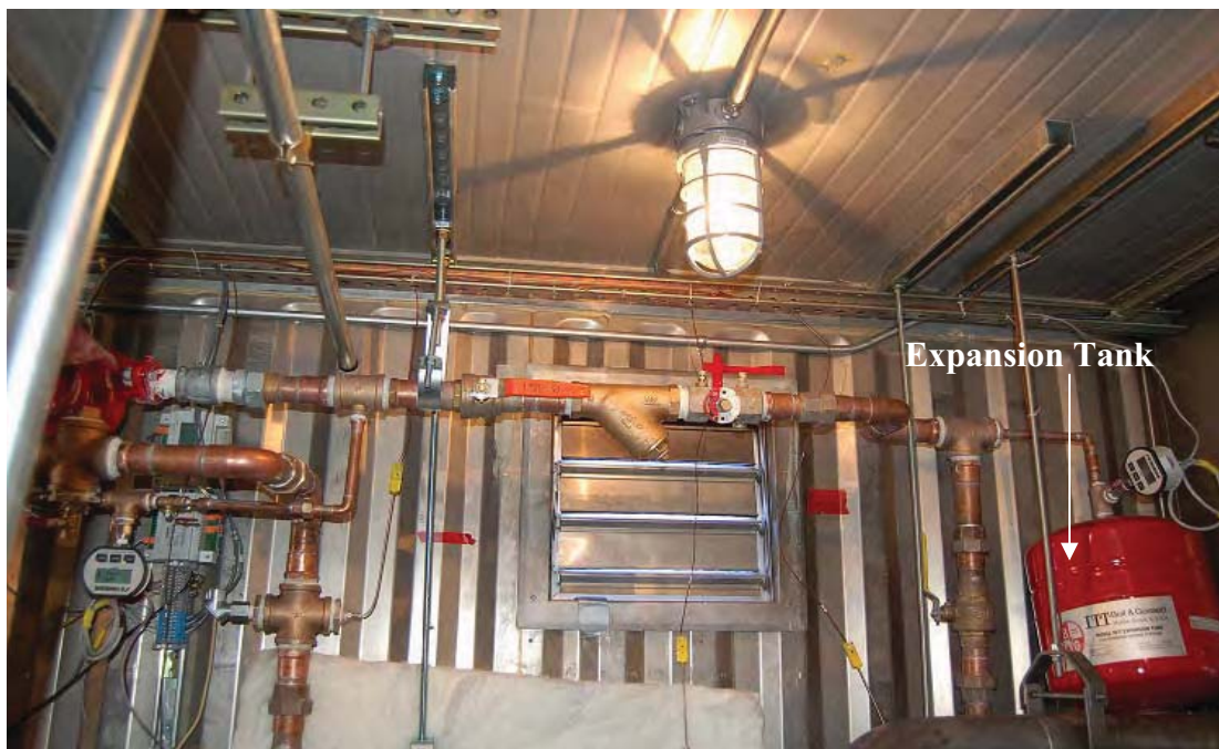
Figure 2.14. Expansion tank in the control system
