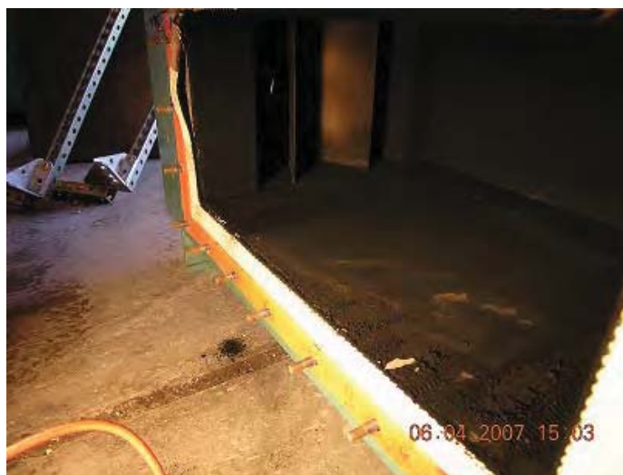
Figure 3.15. Shell side soot accumulation.
