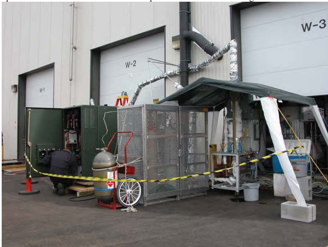
Figure 3 Setup in the parking lot at INEEL. Acumentrics fuel cell at left, SOFCo reformer at right. Natural gas supply in tank with wheels, the insulated line at the top is for the steam supply.
