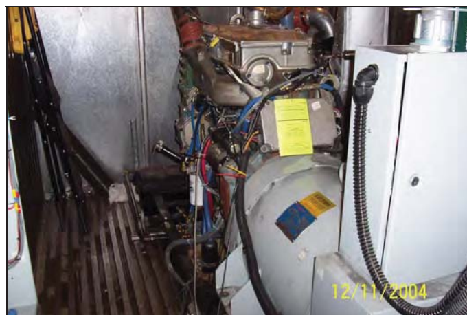
Figure 3.1: Diesel Electric Generator (125 kWe Detroit Diesel) at UAF Energy Center.
