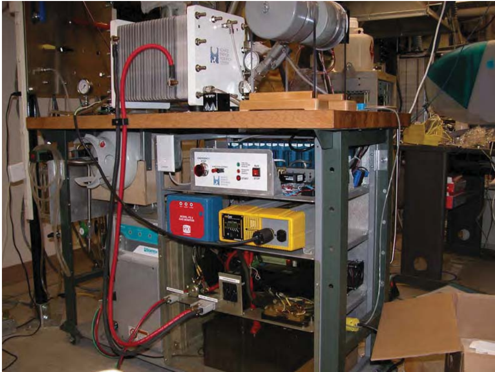
Figure 6 Front view of integrated system. Reformer, hydrogen ballast, batteries, inverter, safety system, and control system are visible.
