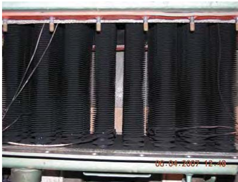
Figure 3.17. Soot accumulation on the core side.
