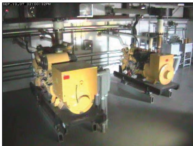
Figure 4.26: CAT ® Diesel Electric Generators at Buckland, AK (455 kWe on left and 175 kWe on right).
