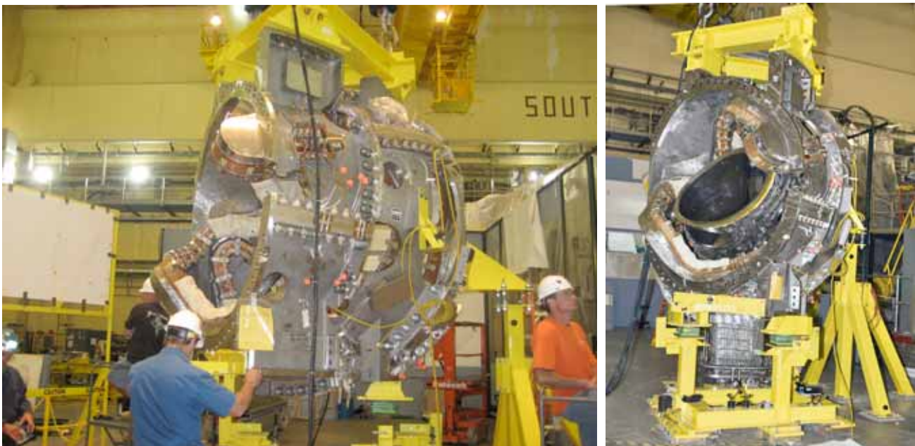
Fig. 12. Modular coil half-period lift and guidance apparatus under test and half-period assembled over vacuum vessel sector.
