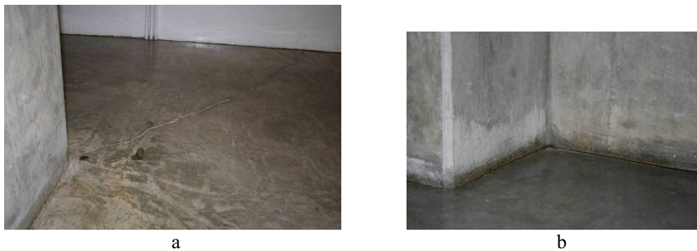
Figure 7. EBR I Reactor Building Basement: a) floor crack, b) stains.
