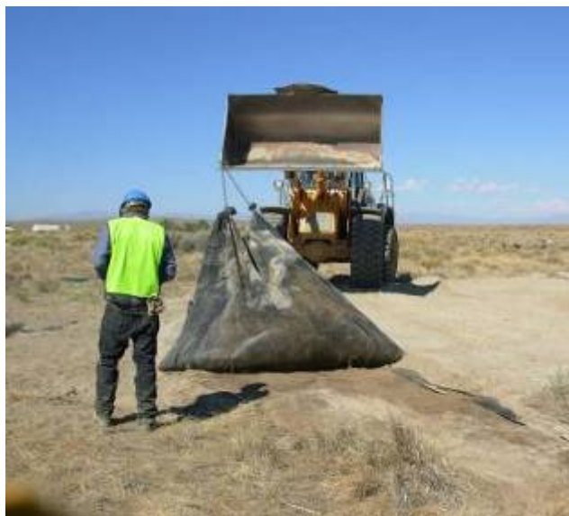
Figure 6. Removal of geotextile fabric from surface at site 10-BT-2189 at the location of the BLR-8 backhoe trench. Note undisturbed surface preserved beneath the fabric.
