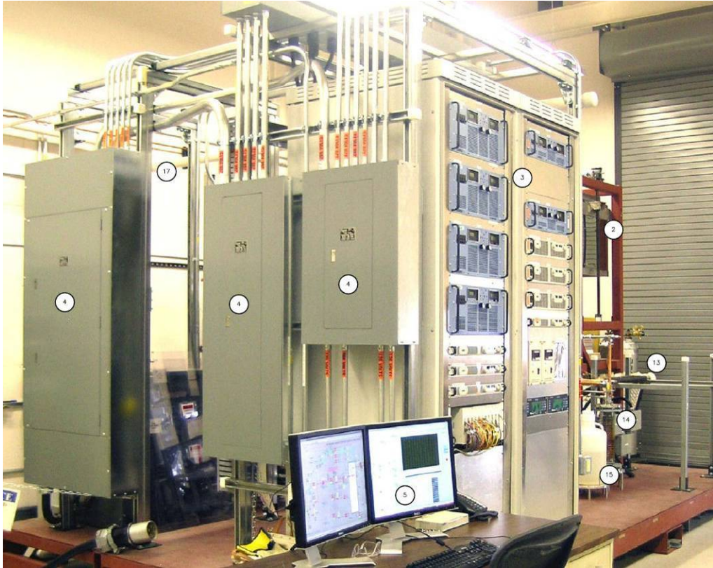
Figure 4. Left side view of INL ILS facility, with major components labeled.
