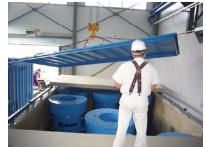
Figure 11. High-Level Waste Storage Facility extension cask storage vault.
