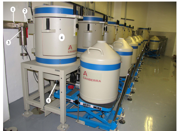
FIGURE 2: The seven FPMS detector stations installed at the Advanced Test Reactor. The pipe chase channel (1) carries the test capsule effluent lines to and from the monitoring stations. Each capsule effluent line (2) branches from the channel, passes through the gross radiation monitoring station (3) where it is viewed by a shielded NaI(Tl) detector, and then into the HPGe spectrometer shield (4) and through the spectrometer sample chamber viewed by the HPGe detector (5) The effluent line returns to the pipe chase channel and leaves the cubicle to the treatment filters and then to the plant ventilation system.
