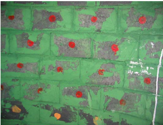
Figure 3. Installation of refractory test panel: arriving at the site (top), and during installation in the side wall of the gasifier (bottom). Test refractory are marked with red dots.
