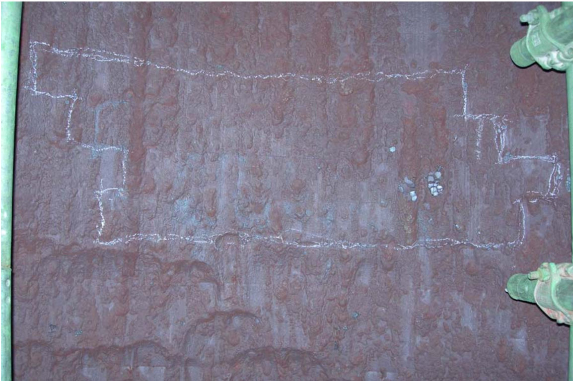
Figure 4. Refractory test panel (approximately outlined with chalk) prior to tear-out following 14 months of service.
