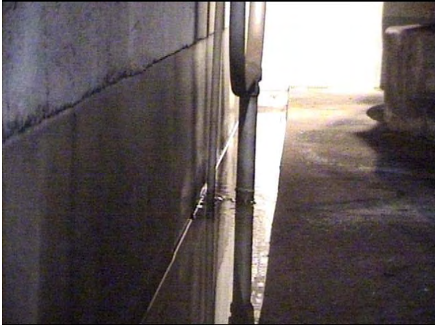
Illustration 13: Trench and Sump as seen by ROV
