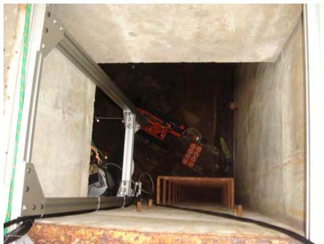
Figure 4.2. Sampling Equipment Installed in Vault
