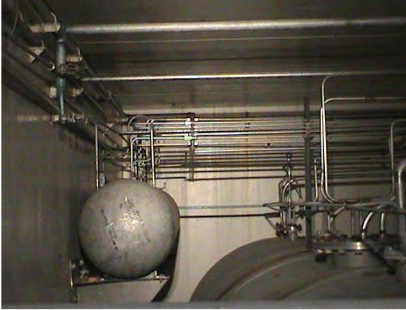
Illustration 41: A-Vault - Tank W-4
