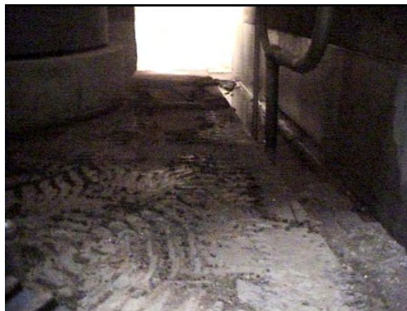
Illustration 10: C-Vault Sump and Trench
