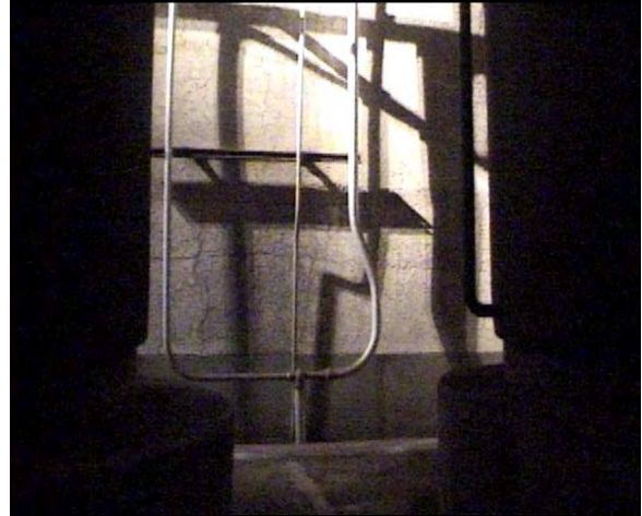
Illustration 20: Sump as Seen From Between Tanks
