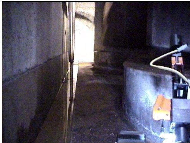
Illustration 12: Trench and Sump as Seen by ROV
