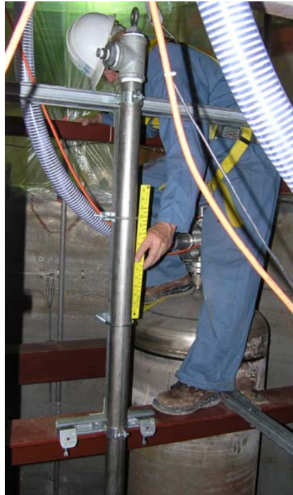
Figure 5.8. The Mount for the Accelerometer Mast
