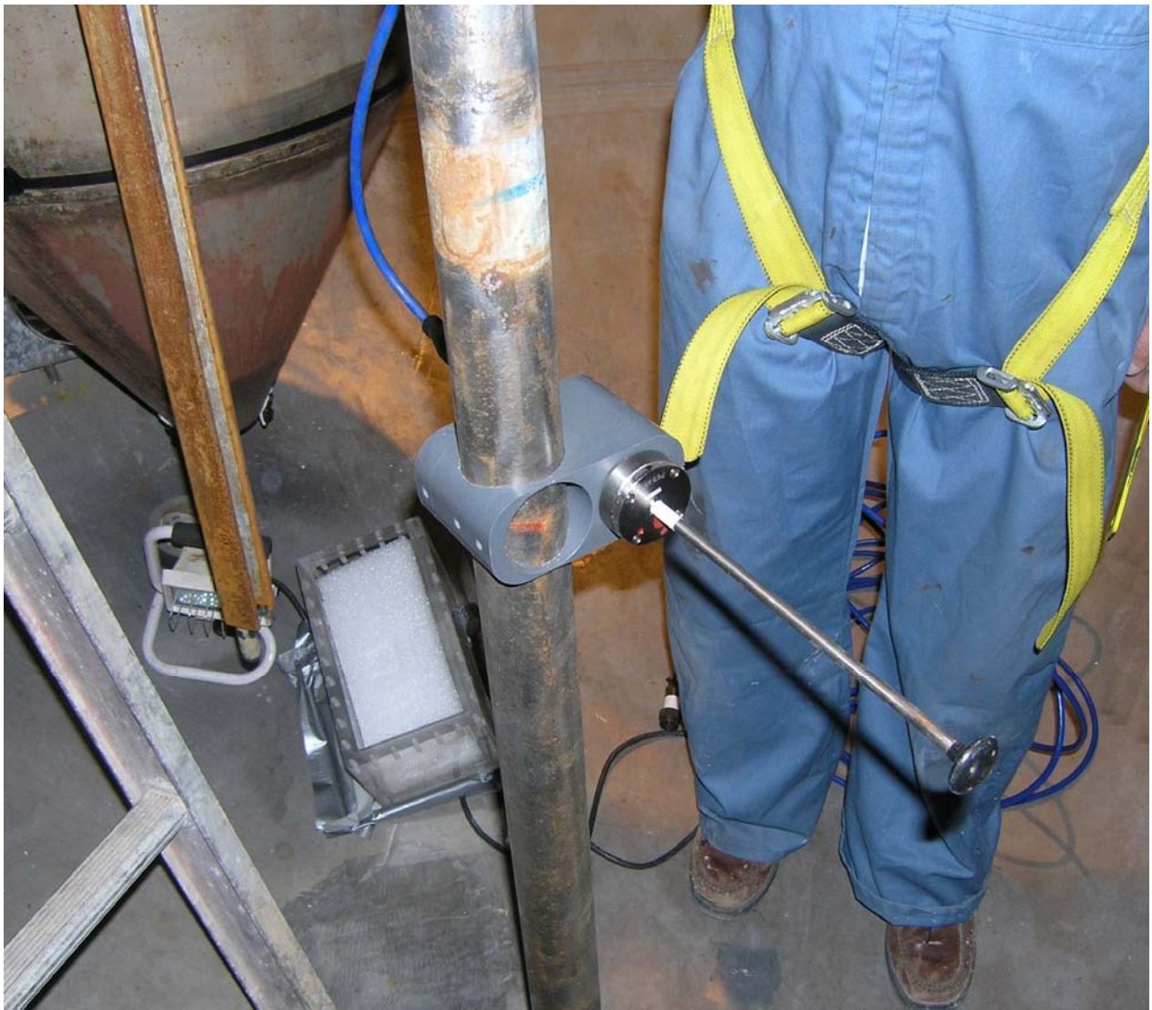
Figure 3.3. Velocity Probe Inside the Tank (in the 4-PJM configuration) at an Early Stage of the Installation. (It is not in the final position.)
