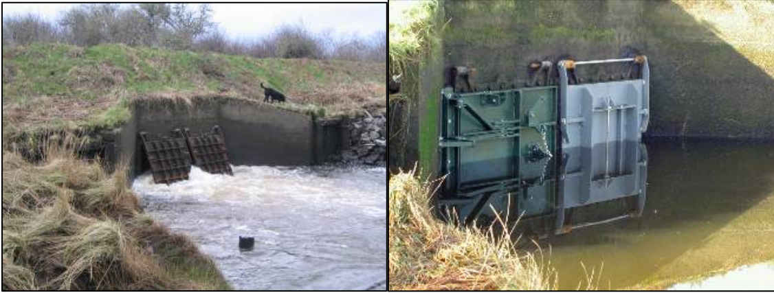
Figure 1.3. Tide Gates at Vera Slough Before (left; open) and After (right; closed) Replacement (photos courtesy of CREST)
