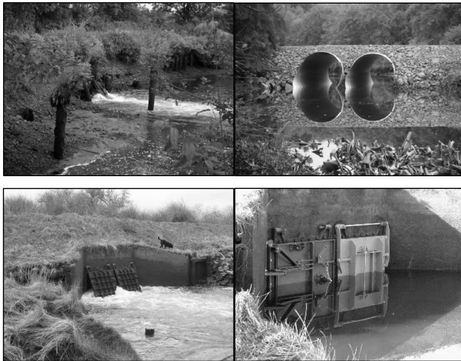
Figure 4.3. Tide Gate with 48-in Culvert on Seal Slough at Kandoll Road (left) Prior to Replacement with Twin, 13-ft Diameter Culverts (right) in 2005 (top) and Tide Gates at Vera Slough before (left) and after (right) Replacement in 2005 (bottom).
