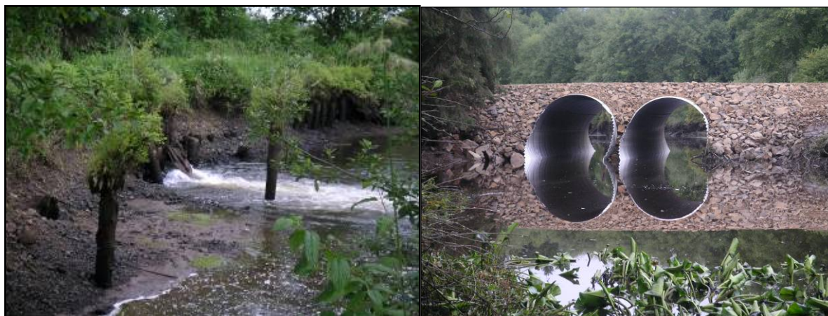
Figure 1.5. Tide Gate at Kandoll Farm before (left) and Culverts after (right) Replacement
