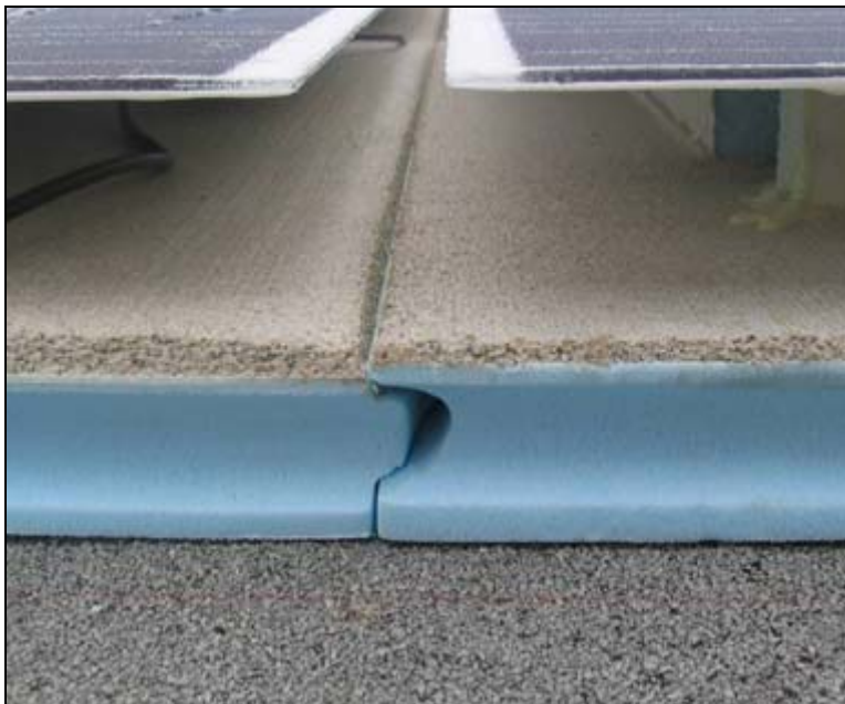
Figure 43: PowerGuard tile with reduced coating thickness (on right).
