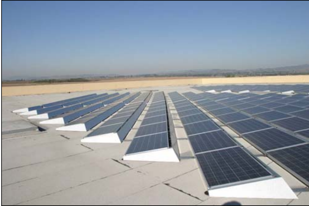
Figure 44: Phase I commercial demonstration project.
