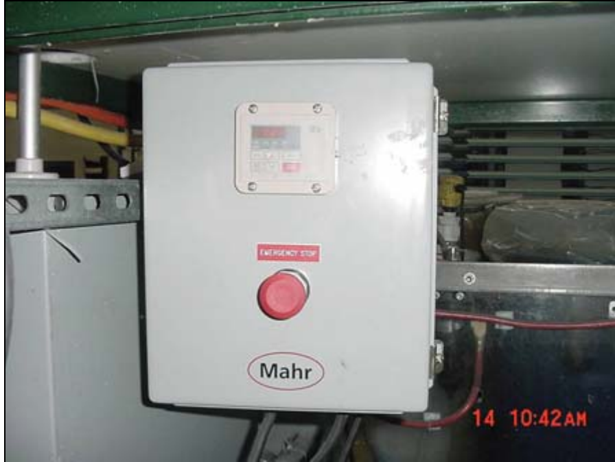
Figure 34: Control panel for pumping station.
