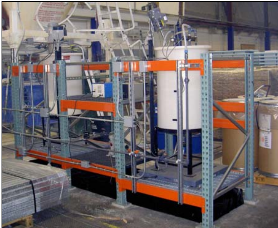
Figure 35: New liquid metering system.
