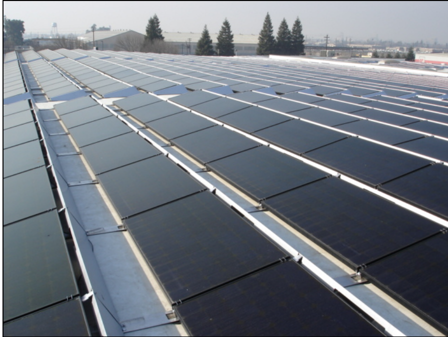
Figure 12: Installed Phase II universal RFT10 system – 1MWp system.
