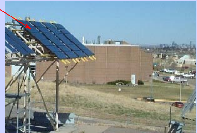
HVST2 array: viewed looking east
