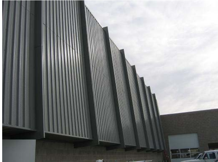
Figure 11 Transpired collector installed on south wall of the Wal-Mart Supercenter in Aurora, Colorado
