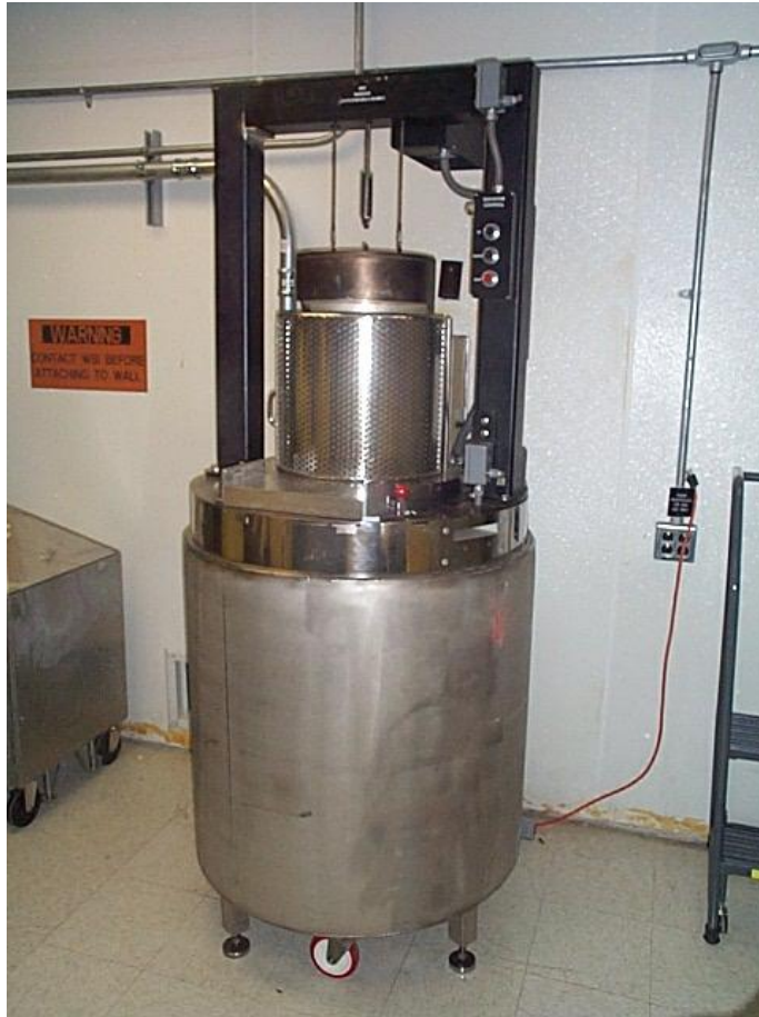
Figure 1. Photo of AWCC installed in HB-Line with chamber open and in the “up” (loading) position.
