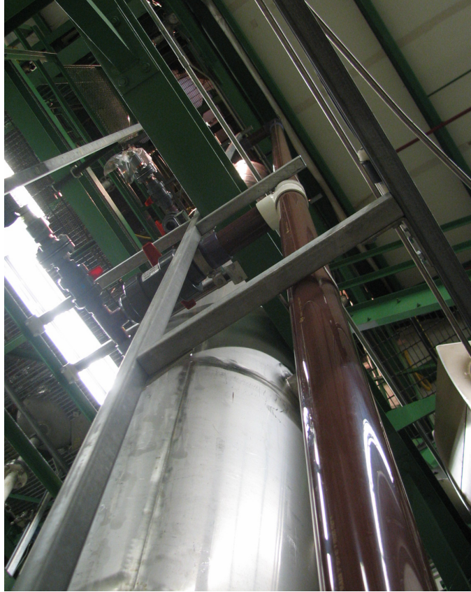
Figure 4: Bubble Column and Transparent External Piping
