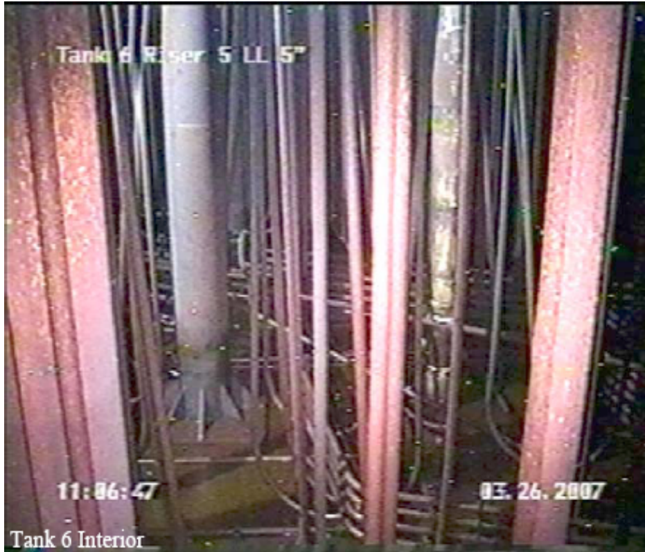
Fig. 1. Tank 6 interior showing numerous cooling coil and equipment interferences.
