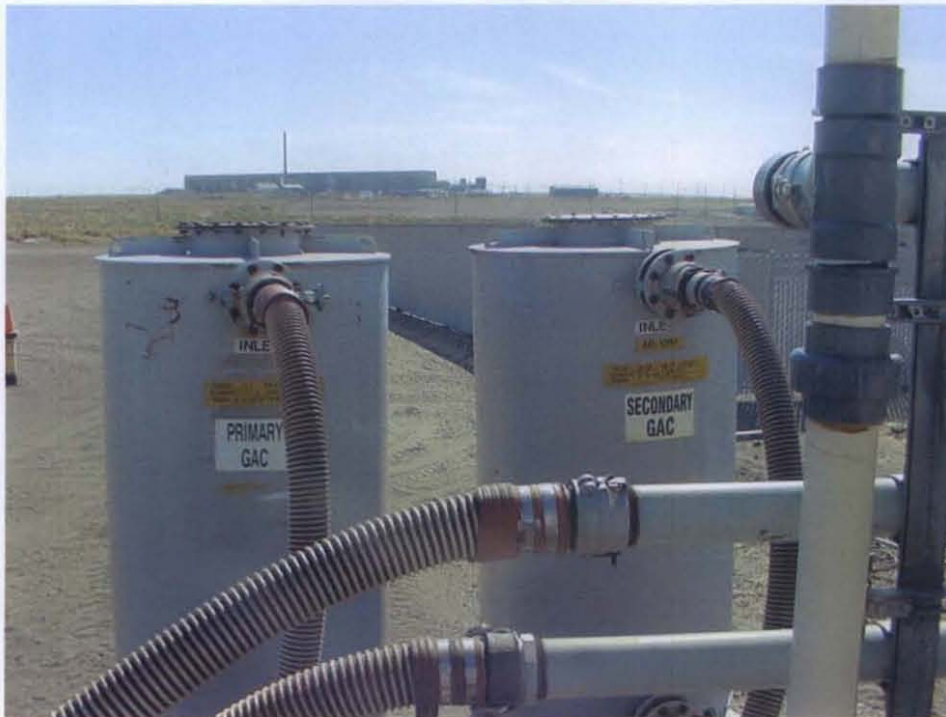
Figure 1-7. 200-PW-1 Granular Activated Carbon Canisters (Two Used in Series).
