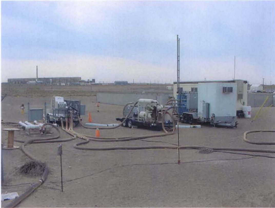
Figure 1-6. 200-PW-1 Soil Vapor Extraction System.
